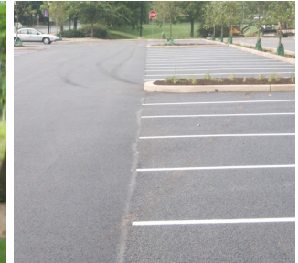
Standard asphalt on left, porous asphalt on right F&M College, Lancaster, PA
